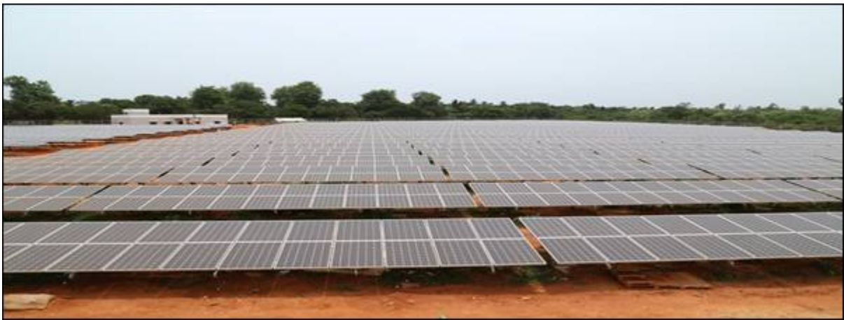
Solar Power Panels at Block-4, Neyveli, NLCIL
