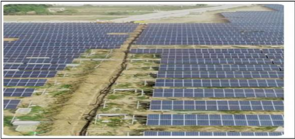
SCCL: Solar Power Plant at Manuguru (30 MW)
